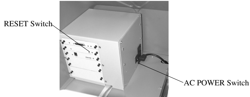
Figure 8-2. The location of the RESET and AC POWER Switch.
